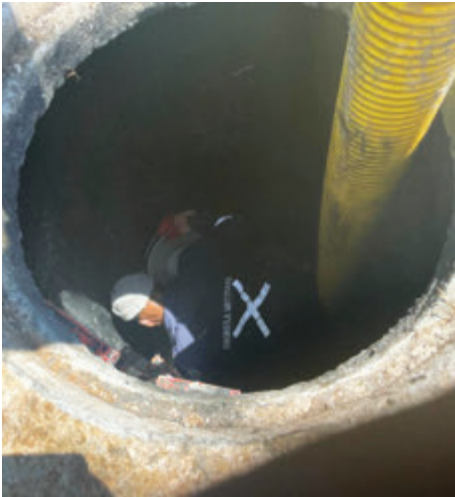
The number of foreign objects in the sewer system is cause for concern.
